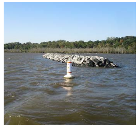
Construction planned for the summer of 2021 will permit the National Park Service to extend the current sill 2,100 feet. Photo by Glenda Booth
