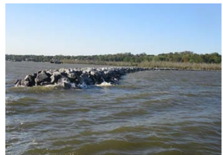
The completed breakwater replicates a protective promontory that dredgers removed. Photo by Glenda Booth
