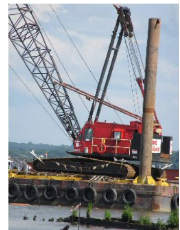
Restoration contractors have brought barges, cranes and boats to work in Dyke Marsh. Photo by Glenda Booth
