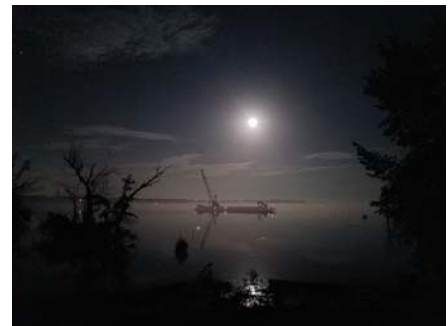
The full moon over Dyke Marsh illuminates a barge and crane, part of restoration activity. Photo by Jim Hutzler
