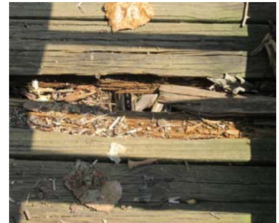
The Dyke Marsh boardwalk is one example of the many maintenance backlog challenges facing NPS. Photo by Glenda Booth
