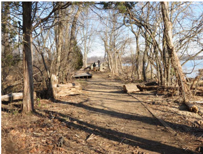
Haul Road trail with damage from a January 2024 storm, flotsam washed up and a displaced ramp to the boardwalk Photo by Stacy Langsdale
